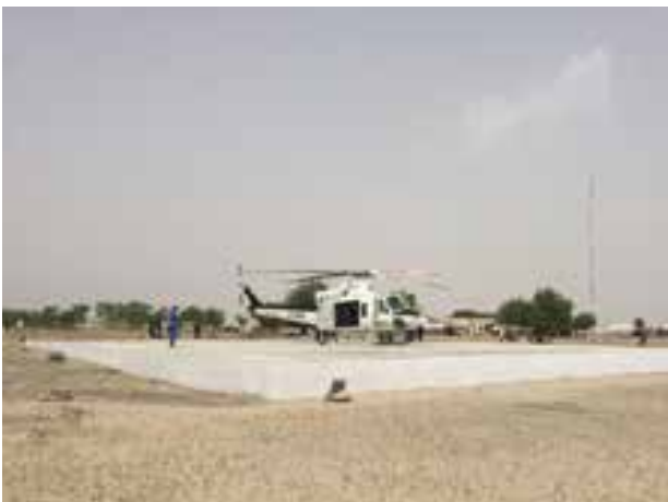
Damboa. Repair works: UNHAS, in conjunction with OXFAM, building a Landing Zone to facilitate transport by helicopter in the area.
