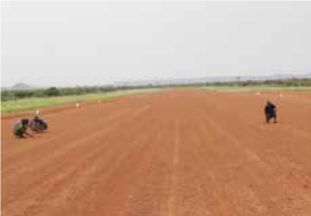
Melkadida airstrip. Repair works: UNHAS staff assisting repair works of cleaning airstrip from grass contamination on the surface.
