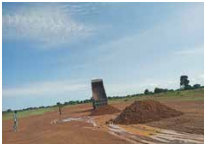
Aweil. Repair works: levelling and compacting the airstrip in coordination with the Aweil State Ministry of infrastructure.
