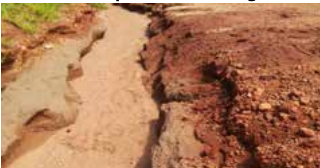
Tshikapa airstrip status in March 2019 before UNHAS repair works.
