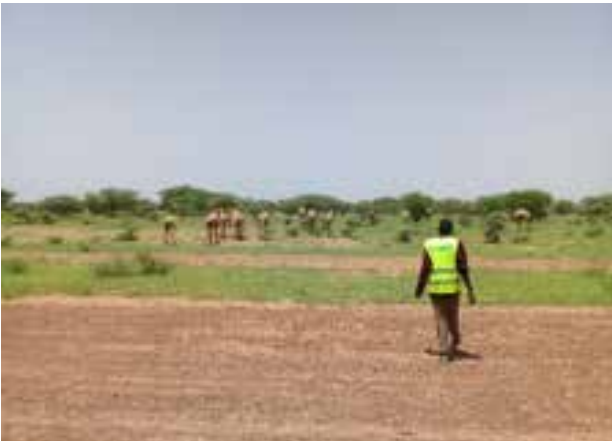
Bassikounou airstrip. Repair works: clearing the runway area from the passage of wild animals.
