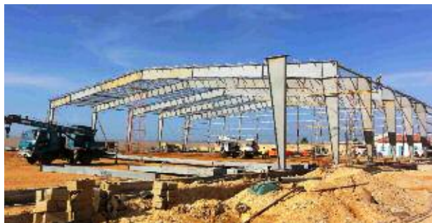
Construction of a WFP warehouse taking place near Port Bossaso in Somalia.
